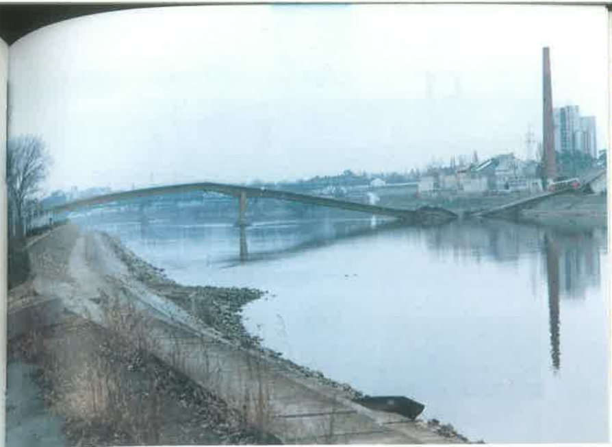
Osijek, collapsed bridge on the river Drava, photo Ivanković
