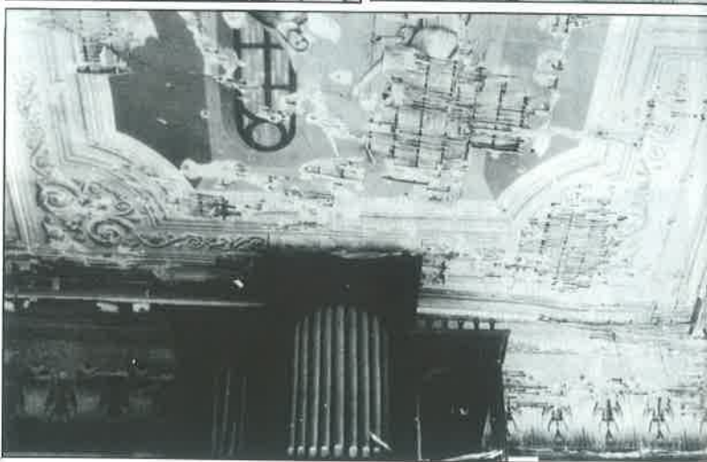
Osijek, Ivanovac, destroyed church
