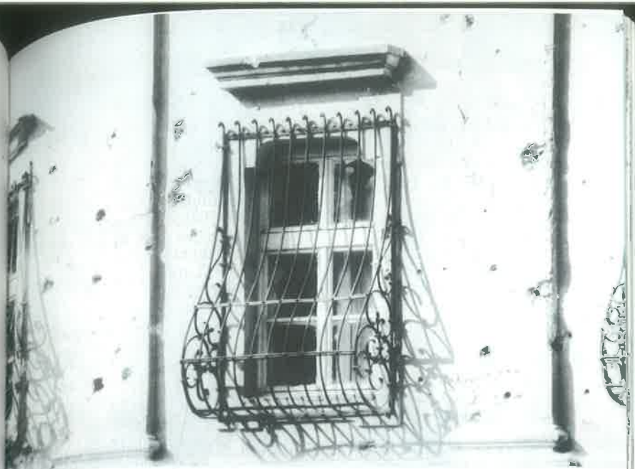
Đakovo, Bishop's court, after damage, photo - personal property
